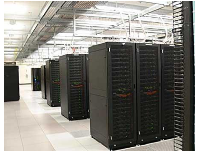
Amazon data center
