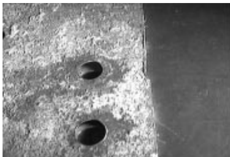
Fig 14a. surface with corrosion
